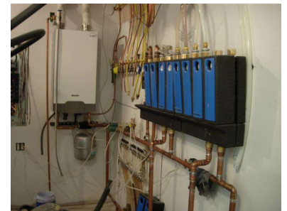
Commercial installation Minnesota
