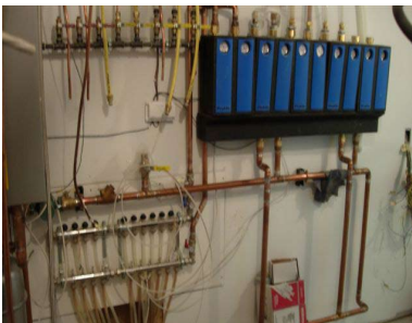
Commercial installation Minnesota
